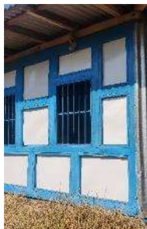
Fig 22: Wooden framed enclosure
